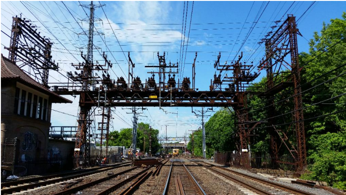
Figure 14. Passenger Railway Supply Substation on the Northeast Corridor.
