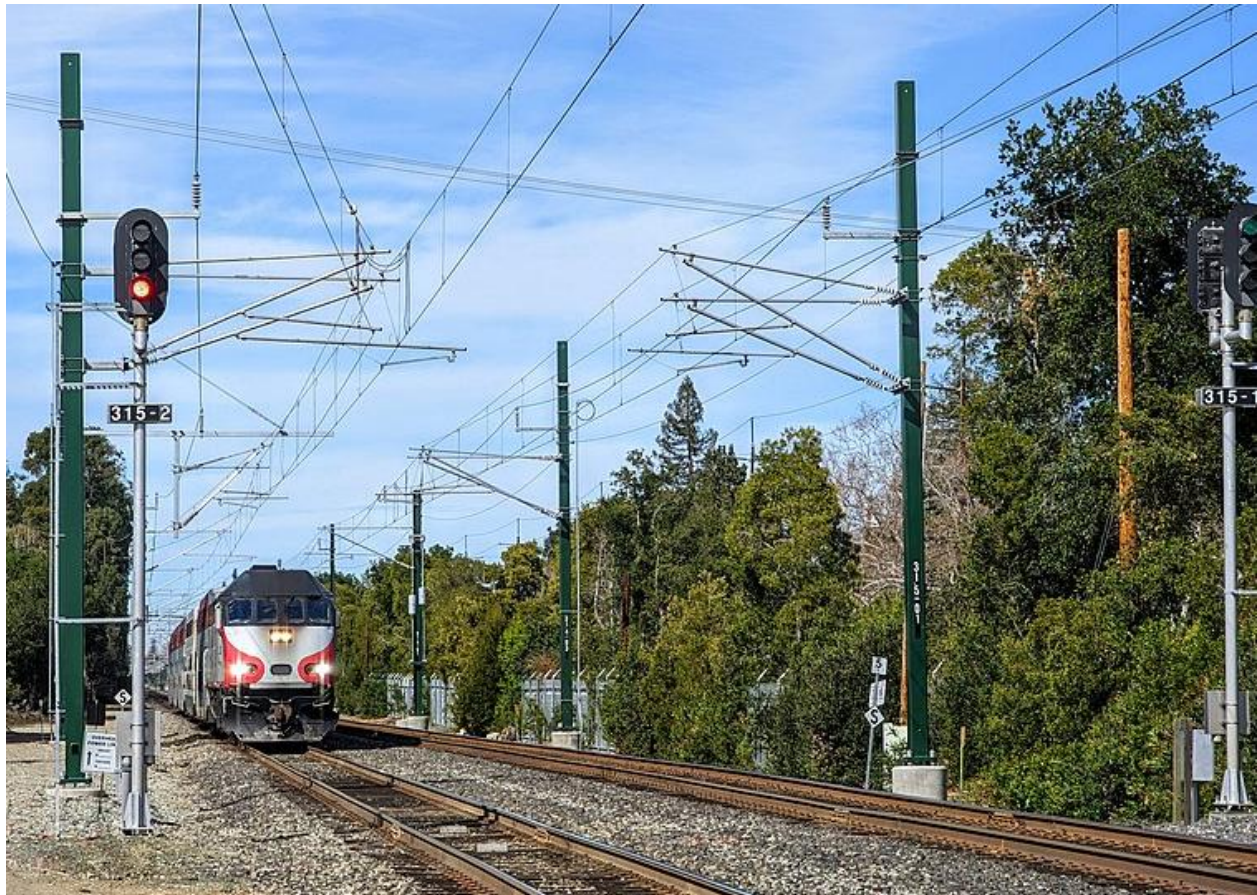
Figure 2. Section of completed Caltrain electrification work at California Avenue, Palo Alto, California, 2022. Dick Lyon photo (CC BY-SA 4.0).
